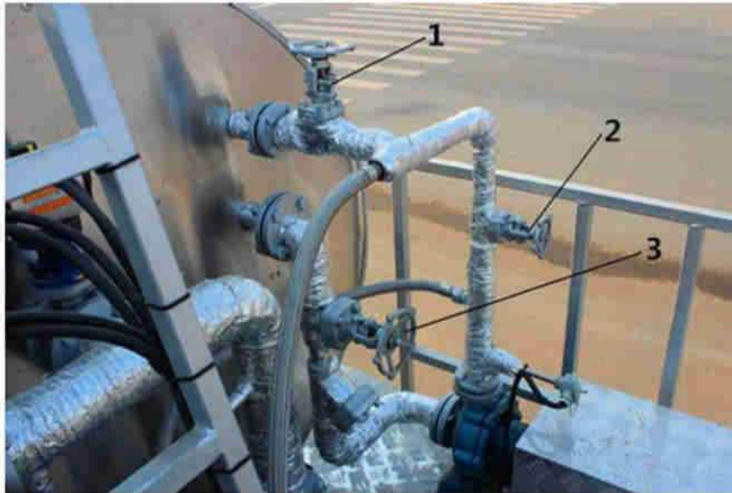
Fig. 11 Heat transfer oil valve
